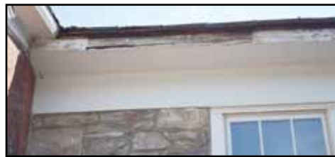
Installing gutters and replacing rotten fascia is needed.
