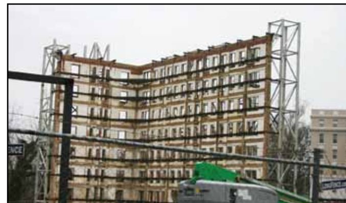
This building in Washington D.C. is currently undergoing a complete renovation to include underground parking.
