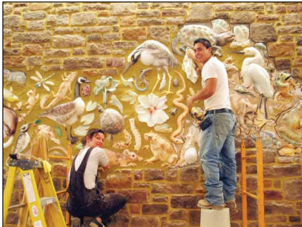
Aimee Curl and Ismael Bonilla helping with the installation of the Gum Springs Library tile wall.
