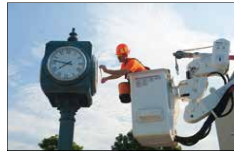
Chad Sager with RCD, Inc. Electrical Services
