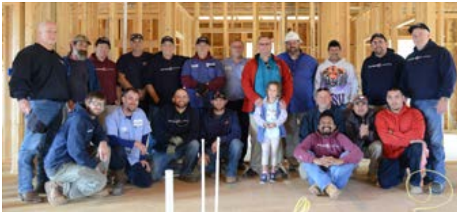
19 Volunteers from Southern Electrical of Leesburg donated their time on a Saturday and wired the house in four hours – pictured here with Sgt. Slease and his daughter.
