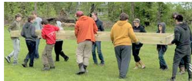
Scouts of Troop 962-B construct a bridge for the Lovettsville Game Club property.
